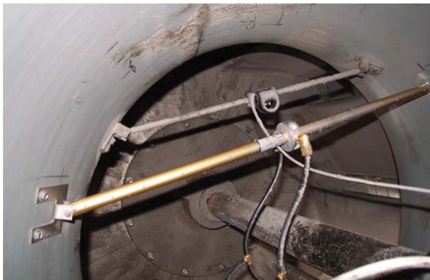
A Pitot-tube sensor (foreground) and a thermal-dispersion device (background).
