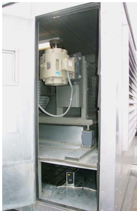
Access to the airflow sensor was limited.
